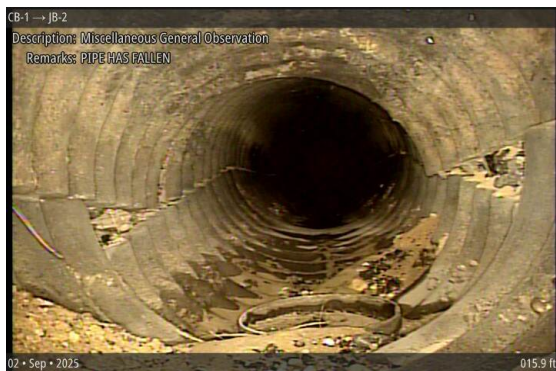
Miscellaneous General Observation at 015.9 ft | PIPE HAS FALLEN
